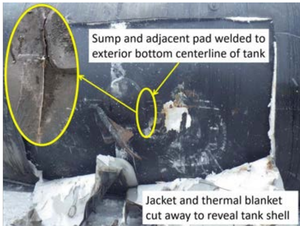
Figure 17 A 12-inch crack initiated between the welds of a sump and adjacent reinforcement pad. The stainless steel jacket had to be cut away to reveal the exterior of the tank shell.
