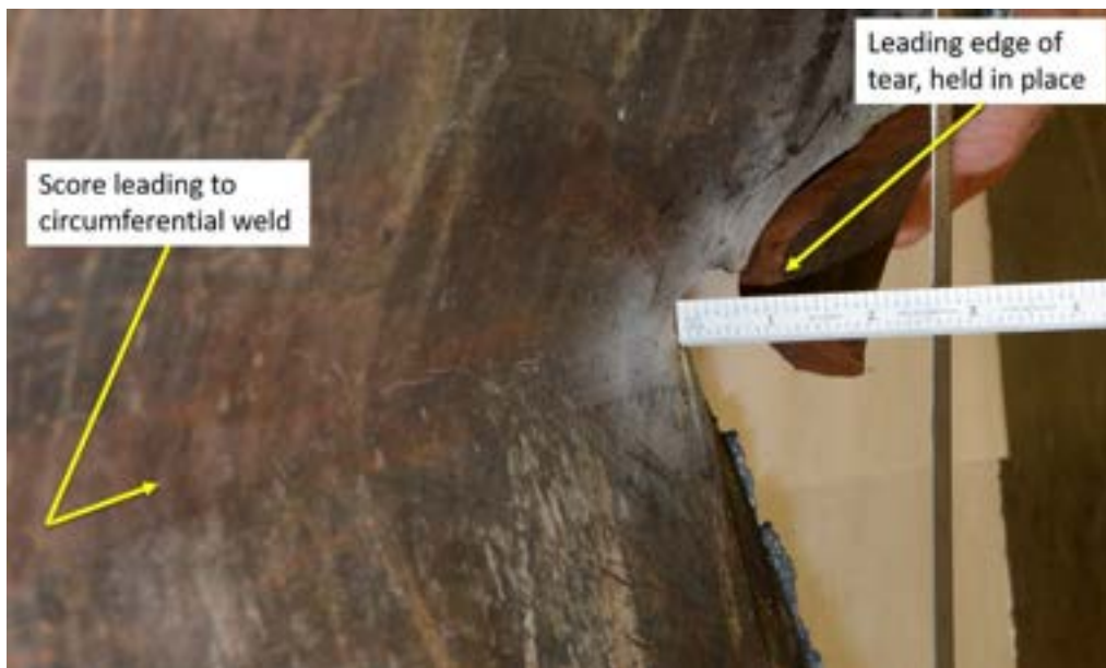
Figure 9 Close-up image of the damage within the oval in Figures 7 and 8; this view is along the length of the tank to illustrate the 2-1/2-inch (plus) depth of the dent that was associated with the score. 11
