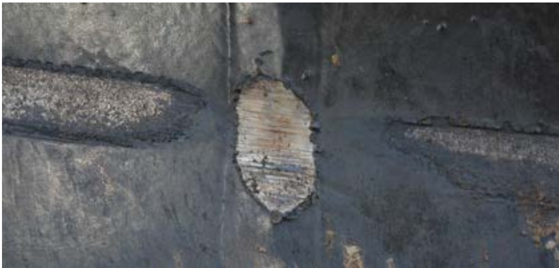
A gouge that removed metal from the crown of a girth weld; the removal of metal that is limited to the crown/reinforcement is not critical.
