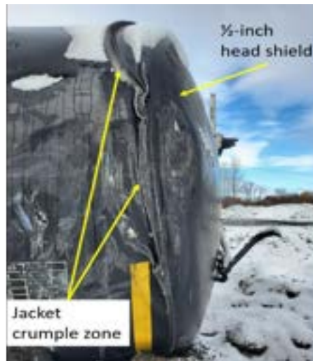
Figure 20 When a head shield is impacted during a derailment, it is pushed back against the tank head, crushing the insulation and thermal blanket, and crumpling the adjacent jacket sheets.
