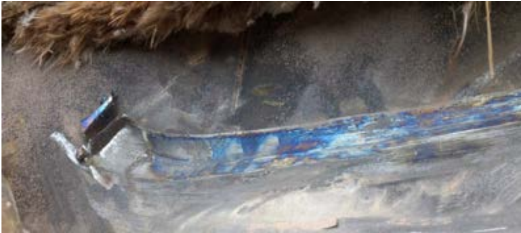
Gouge and rail burn in tank shell.
