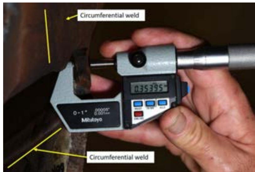
Figure 11 Measurement of the tank shell immediately adjacent to where the circumferential weld began to tear away; refer to the area identified by the blue arrow in Figure 10 above. 13
